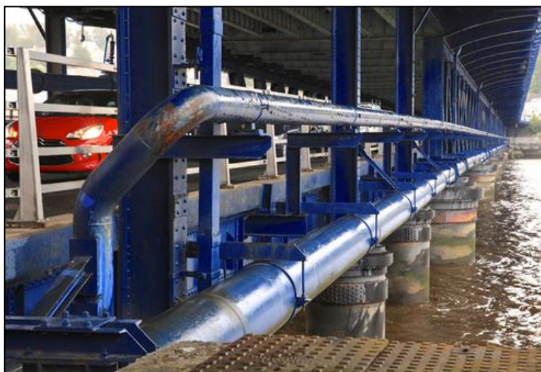
Figure 11.5a: Craigavon Bridge pipeline with evidence of corrosion
